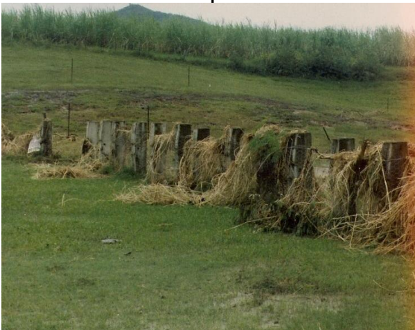
Debris caught on sleepers
